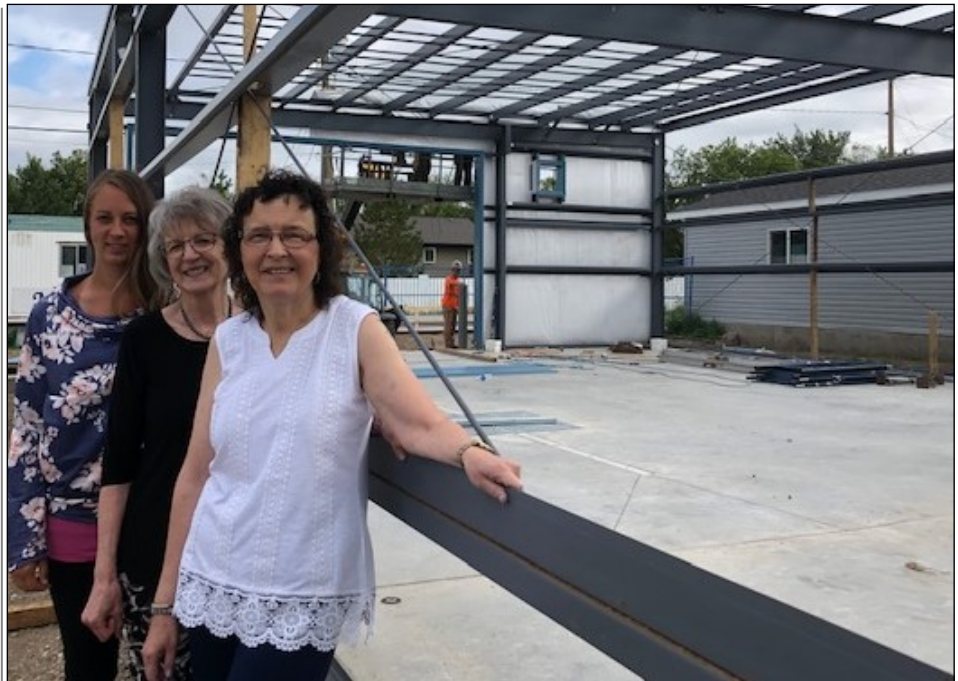
Dundurn Rural Water Utility office staff (L to R) Chantel Hendry, Barb Olyniuk and Ros Arndt are excited about the new building and patiently await for it to be completed.
